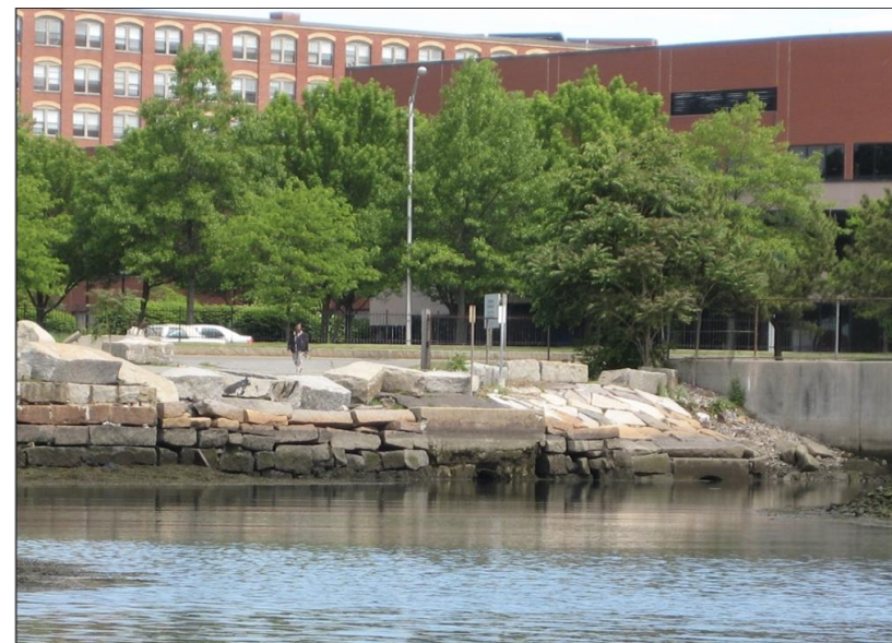
Box culvert at head of Lynn Harbor at mid-tide on 03 June 2009. View looks north.
