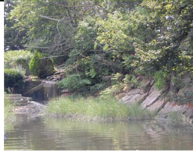
Culvert (note bars covering opening) on Northeast side of MA 103/Wilbur Ave. Bridge
