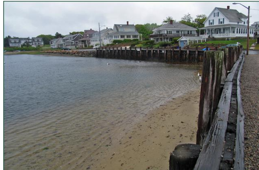
Seawall inside Wild Harbor at low tide on 01 Jun 2004. (RPI photo)
