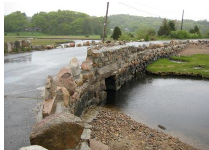
Site of CB-02a and entrance to Wolf Trap Marsh at Ocean St looking north at mid-tide (27 May 2009 photo)
