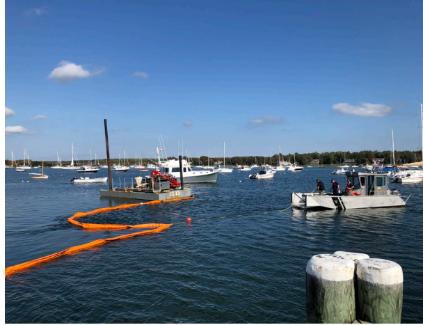
The on-water team tows an anchor system to set the containment strategy around the dredge
